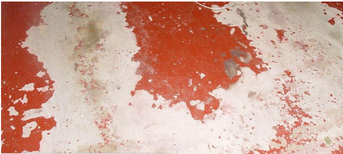
Unsanitary floors with remains of failed concrete coatings.
